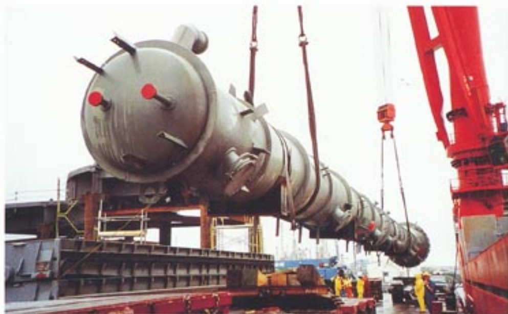
Five distillation columns
